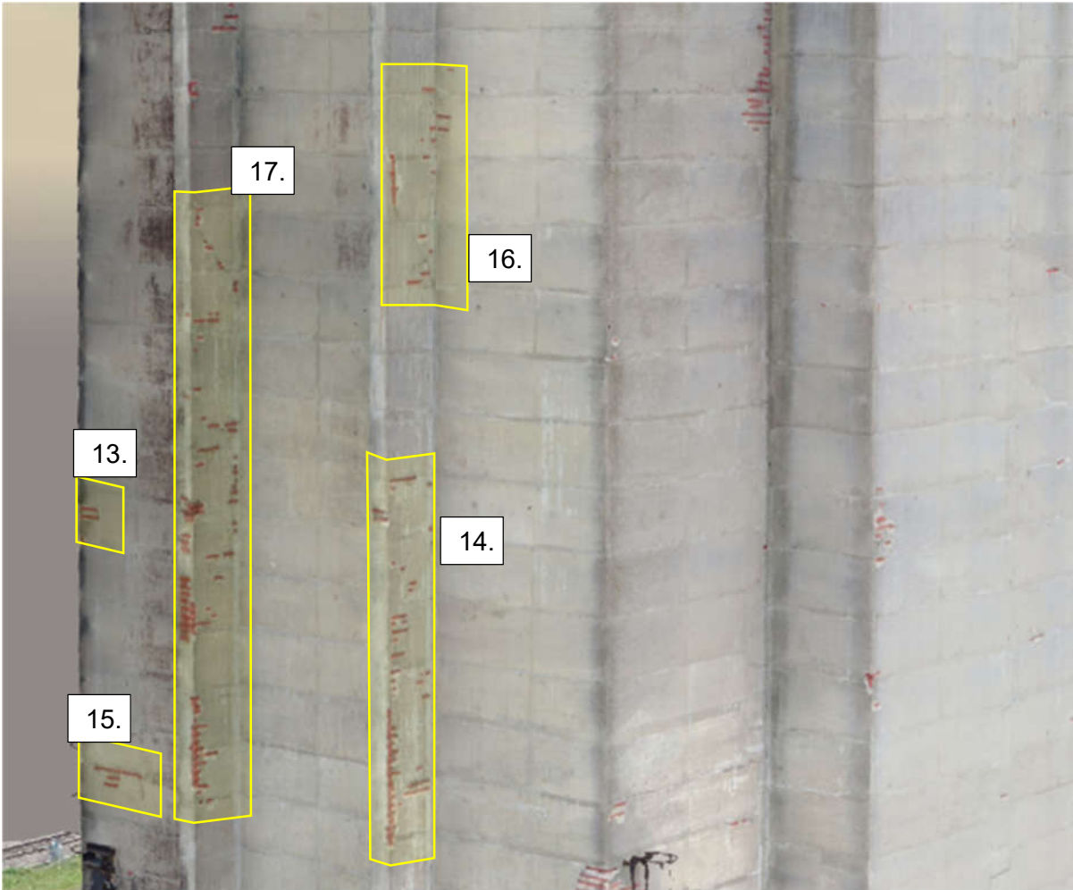
Figure 16: East Elevation - Defects 13-17
