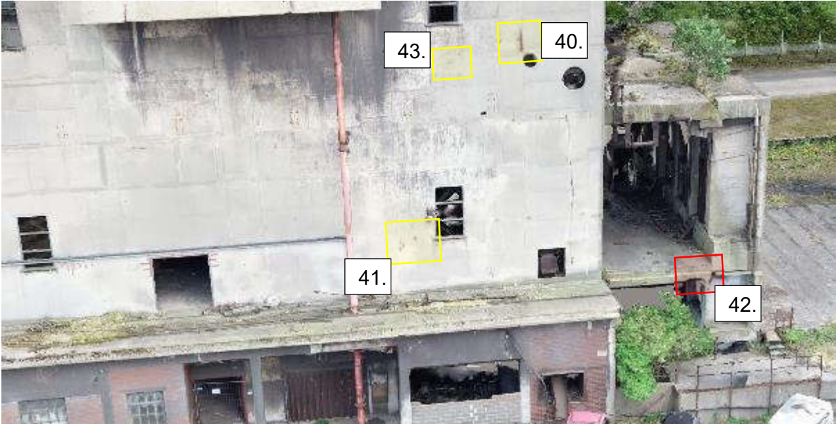
Figure 10: North Elevation - Defects 40-43
