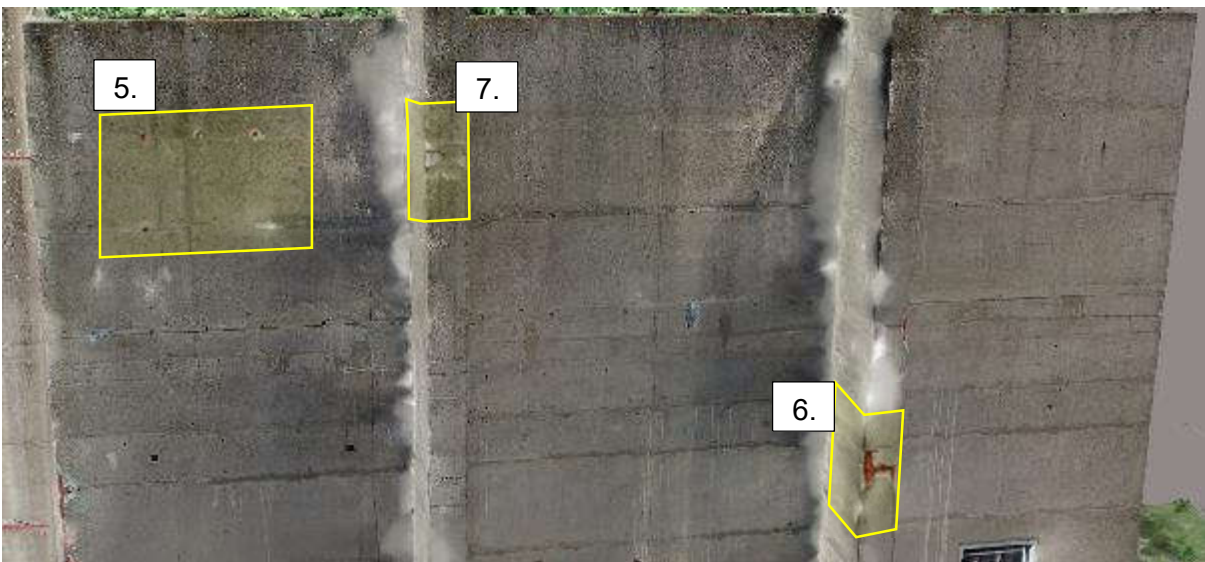
Figure 36: West Elevation - Defects 5-7
