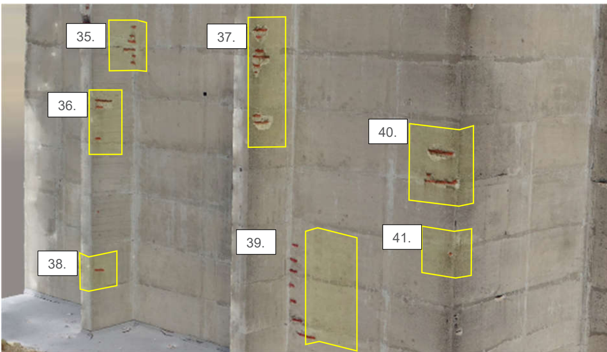
Figure 42: West Elevation - Defects 35-41
