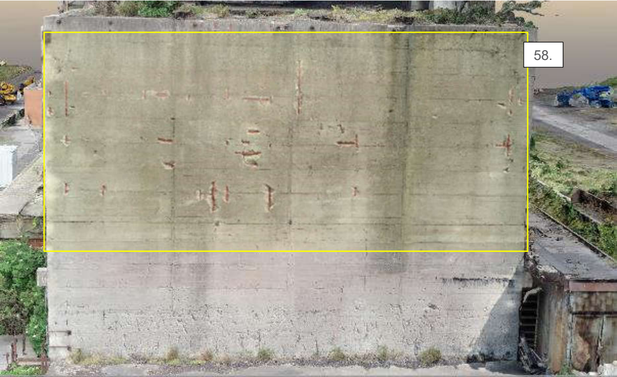
Figure 45: West Elevation - Defect 58
