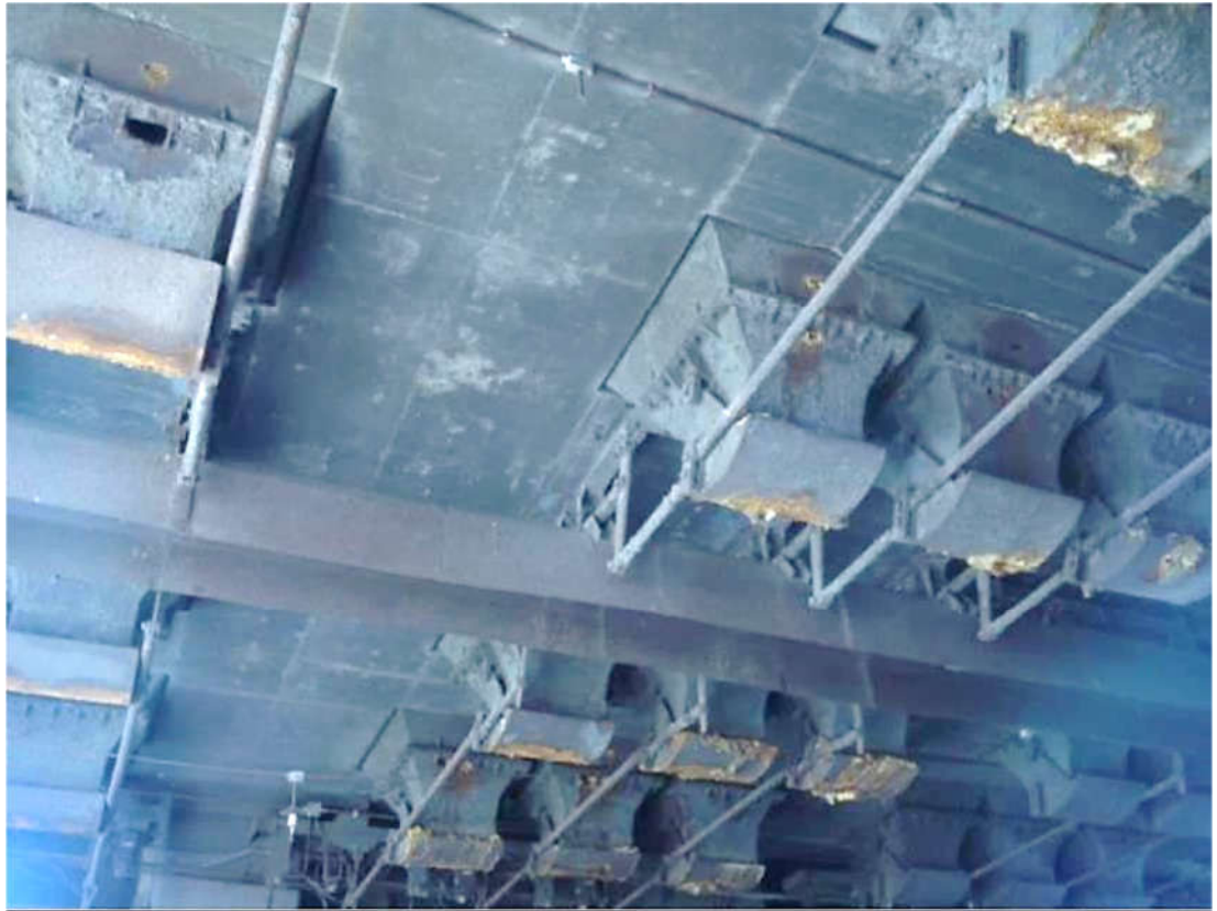
10 3 rd Floor Overhead Bunker Chutes
