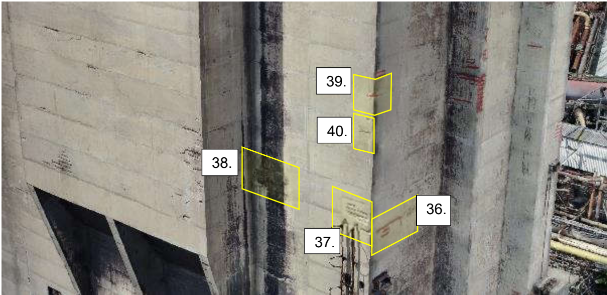
Figure 31: South Elevation - Defects 36-40
