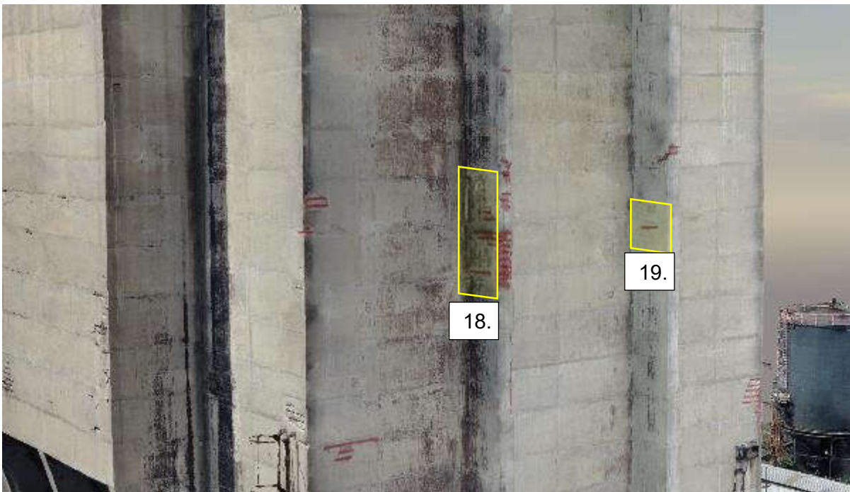
Figure 17: East Elevation - Defects 18-19
