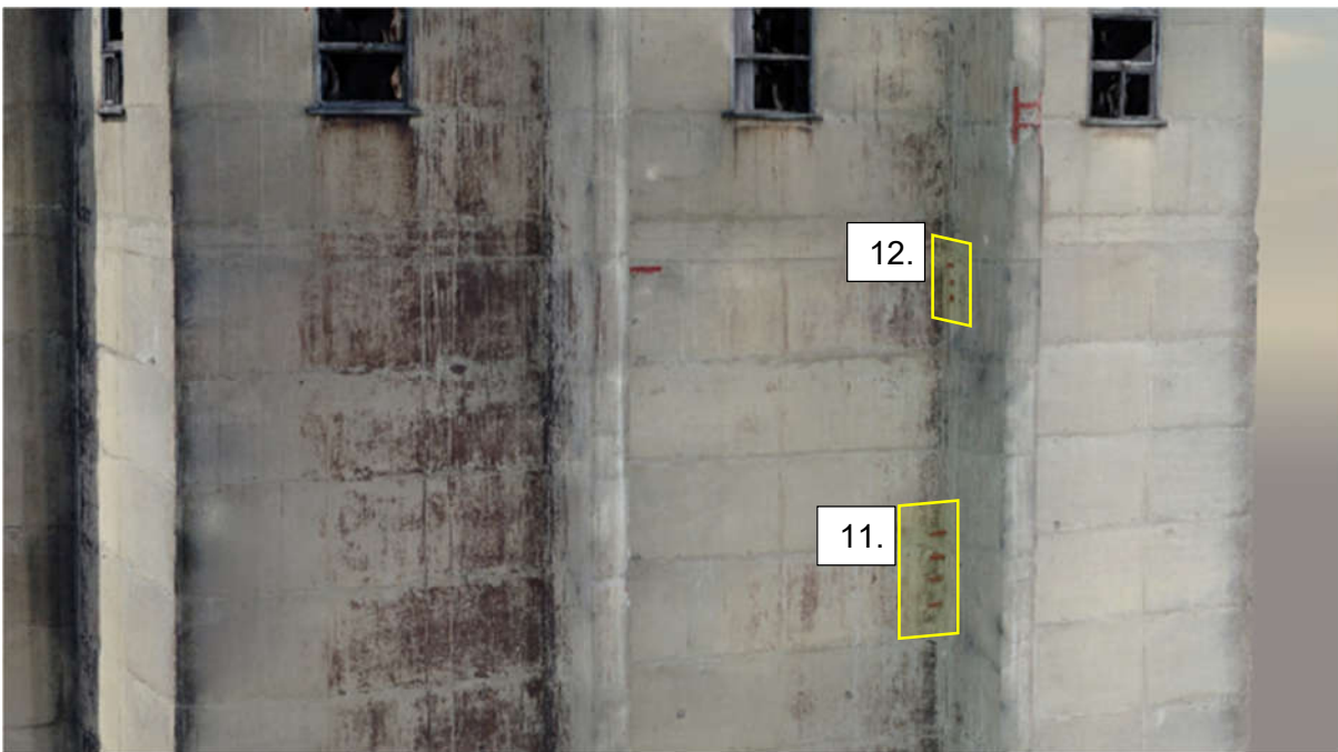
Figure 15: East Elevation - Defects 11-12
