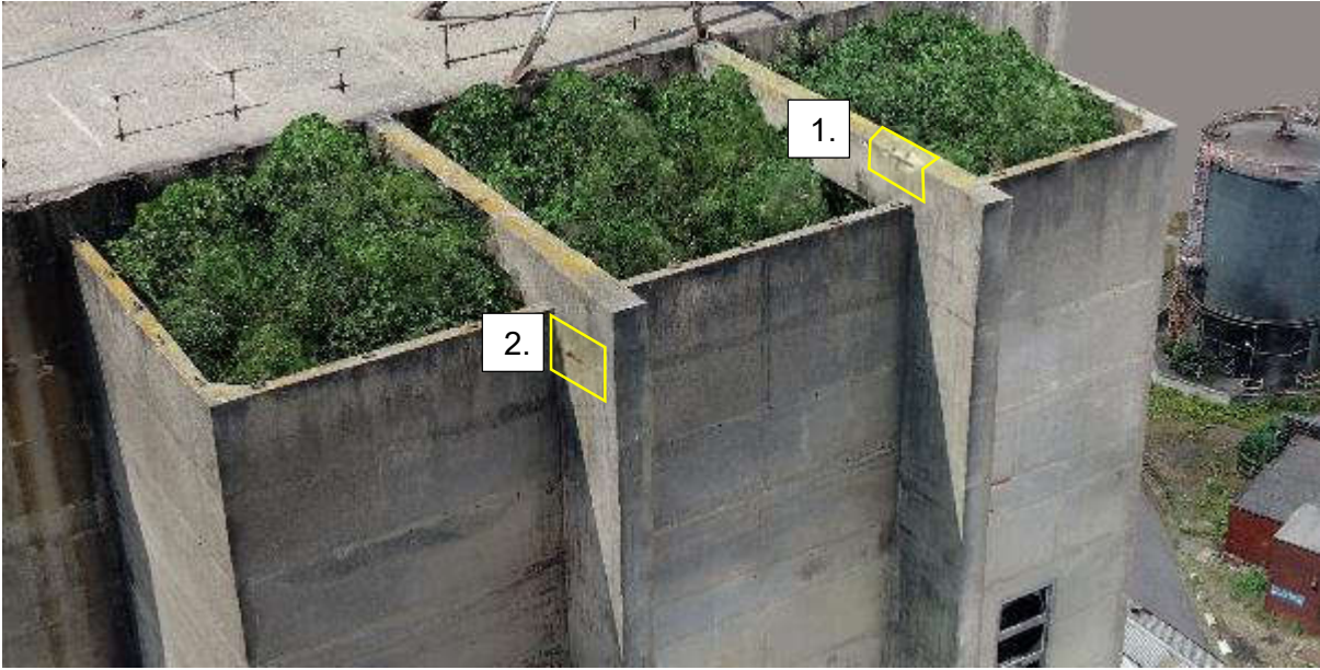
Figure 12: East Elevation - Defects 1-2
