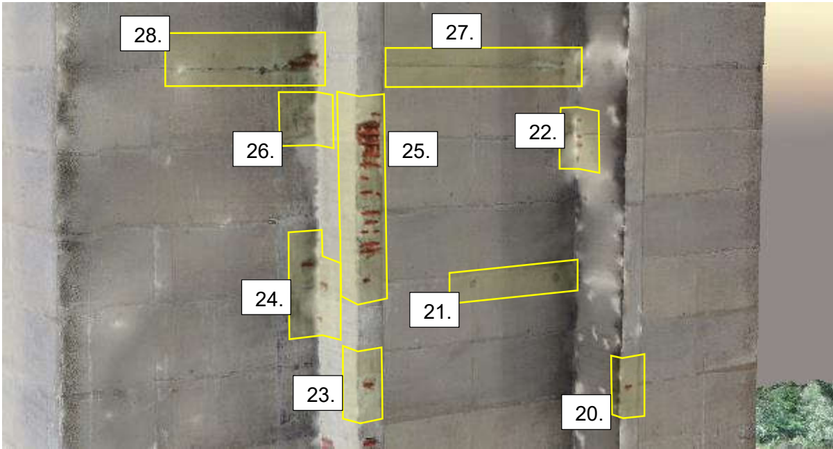
Figure 39: West Elevation - Defects 20-28
