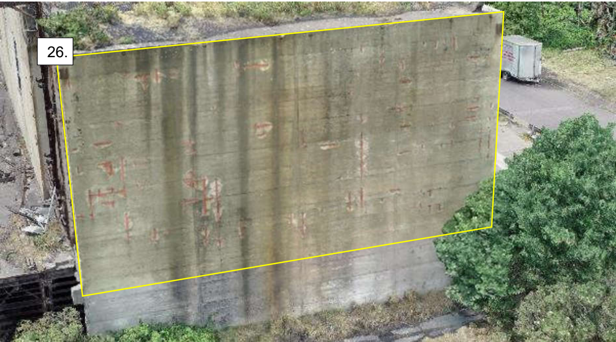
Figure 21: East Elevation - Defect 26
