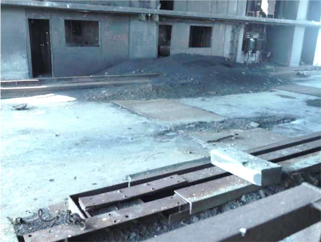
9 3 rd Floor Top Battery Level, below Bunker
